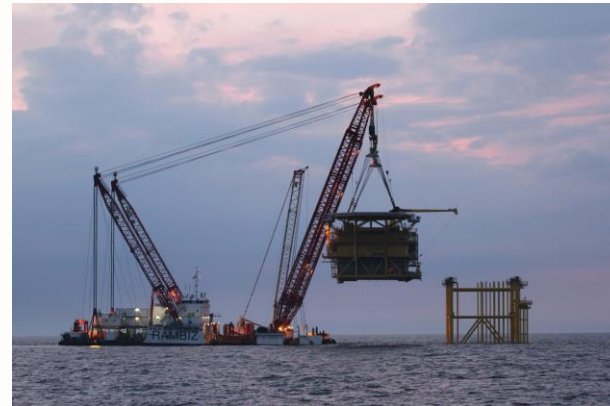
Source: Deme (Butendiek – 288 MW)
